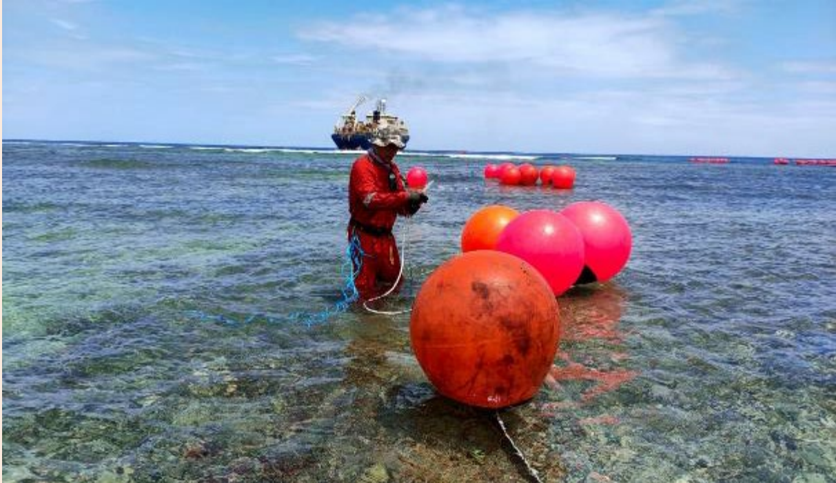
Landing Tokelau's first international subsea cable onto Atafu, Tokelau's northernmost atoll. The international cable went live in September 2023 across all three atolls, with services operated by Teletok, Tokelau's telecommunications provider. Tokelauan communities now have significantly improved international and inter-atoll internet connectivity at a lower cost, and with greater availability and reliability. Credit: McCann Consulting Ltd, 2022
