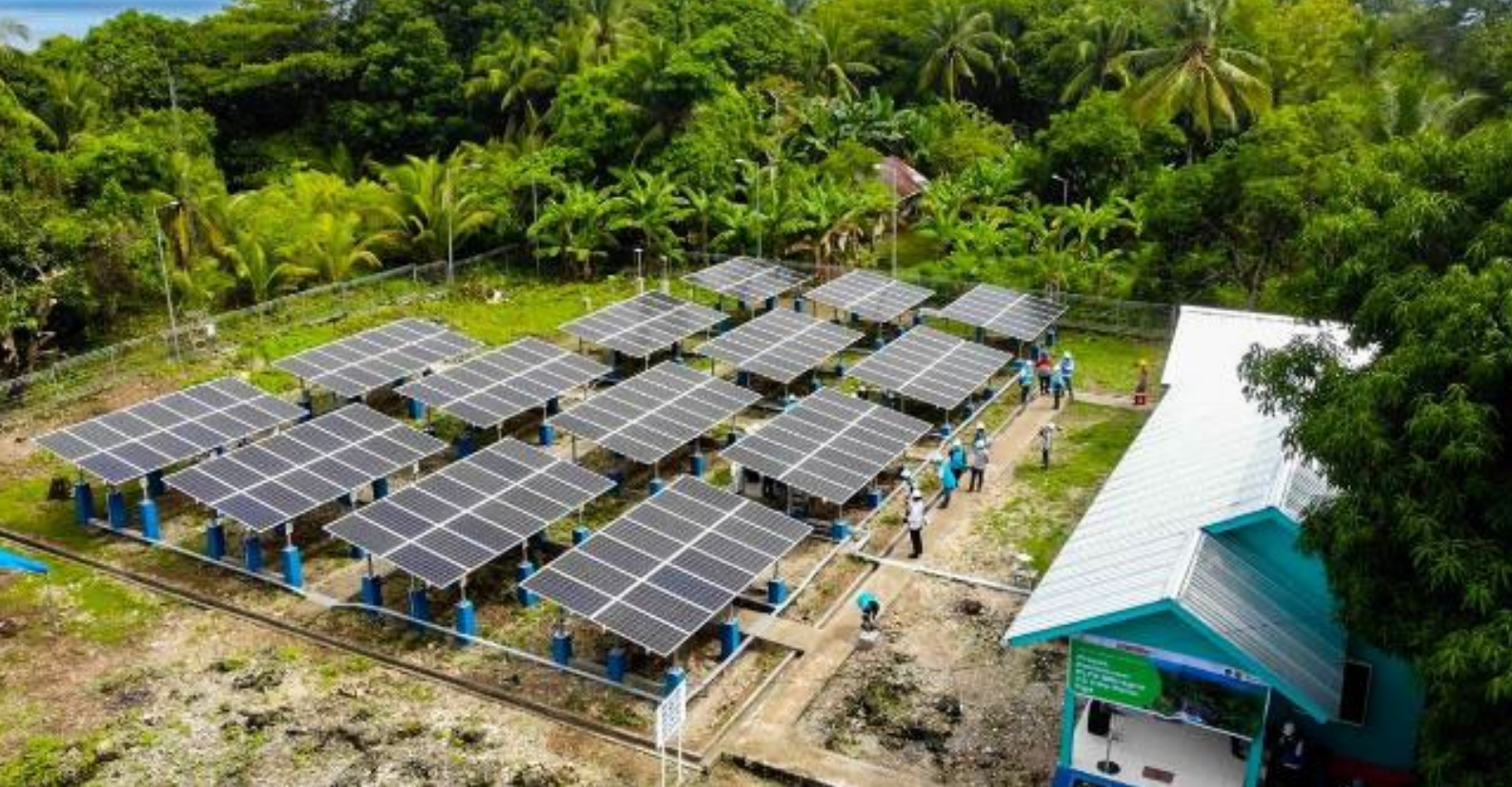
Aerial view of a solar panel installation at Pulau Tiga, Maluku Province, Indonesia. The Access to Renewable Energy in Maluku (NZMATES) programme is in its final year and has seen 1,364 people benefit from improvements to renewable energy infrastructure, and 194 people benefit from training and capability building. Credit: TVRI Ambon Station, Maluku
