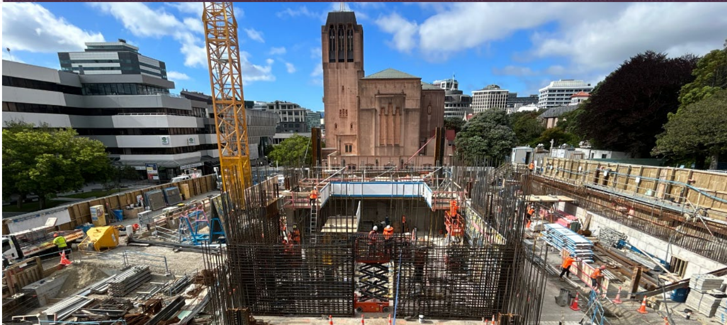
The Ministry's new head office building progress. Credit: Precinct Properties New Zealand Limited.
