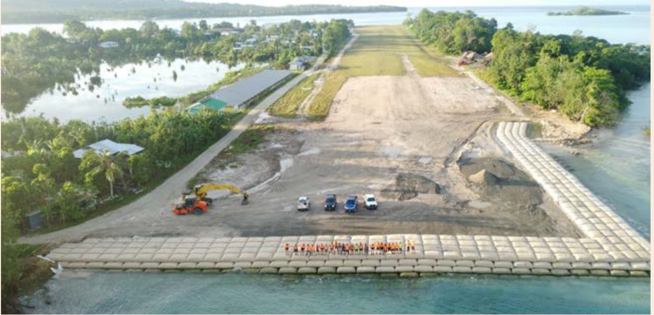
Taro Island, Choiseul Airport seawall construction as part of Solomon Islands Provincial Airfields Upgrade. The team shown is primarily local workers who are engaged and trained by Downers as part of the Ministry's commitment to leave a legacy behind in trained staff, and to provide local employment. 80% of all staff on this project are locally resourced. Credit: Downer Group.
