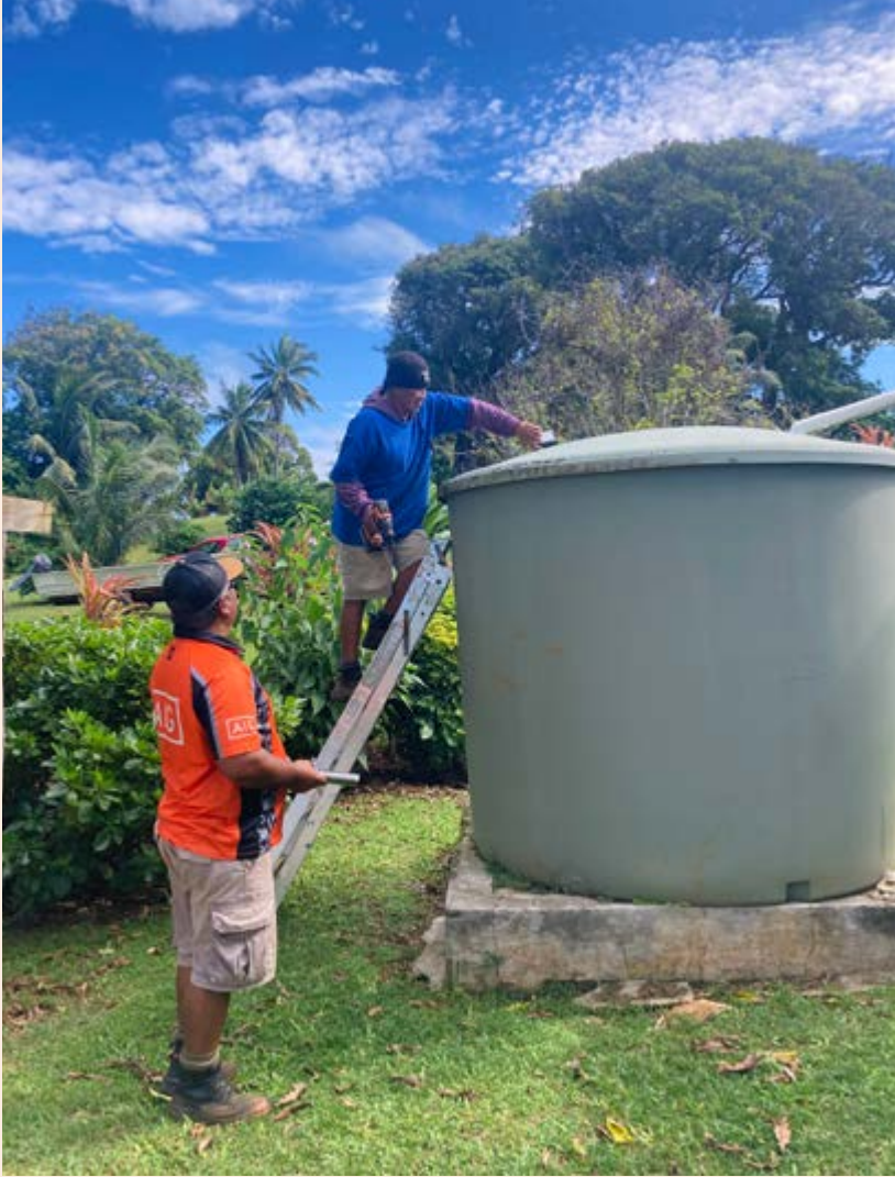
Kaitai Kaitai and Tukua Upokomanu from the Aitutaki Island Government Water Works Department installing the smart sensors. Credit: Engineers Without Borders New Zealand.
