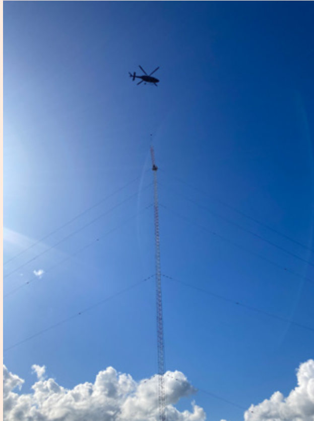
In November 2022, Manatū Taonga and the National Emergency Management Agency announced a $1.48 million package to fund the repair and replacement of three transmission masts in Northland to ensure AM radio could stay on air in the region. Radio transmission proved essential in the area in the aftermath of Cyclone Gabrielle, when power and cellphone signals were affected. Photo: RNZ. Steve White
