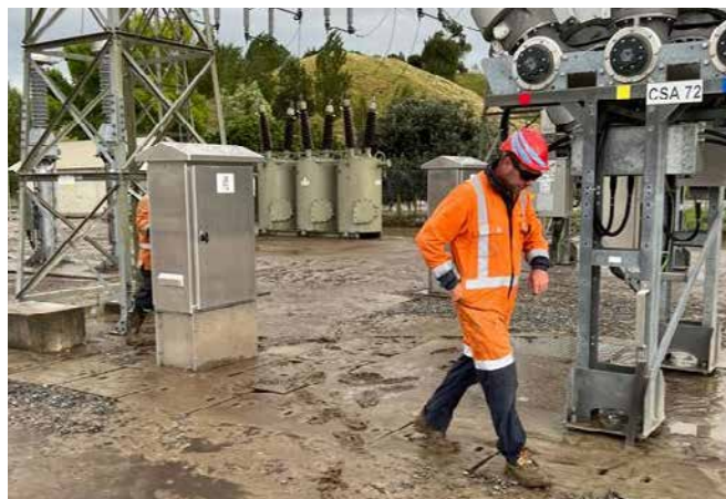
Pictured: Ventia fieldworker at a substation, Hawkes Bay (NZ)
