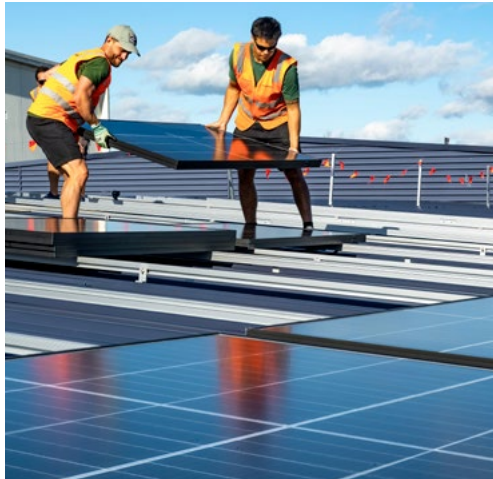
– Solar installation at 3-5 Niall Burgess Road.
