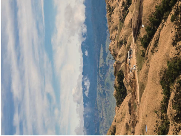
Construction at of Meridian's south wind farm, Harapaki, in the Hauraki Bay.
