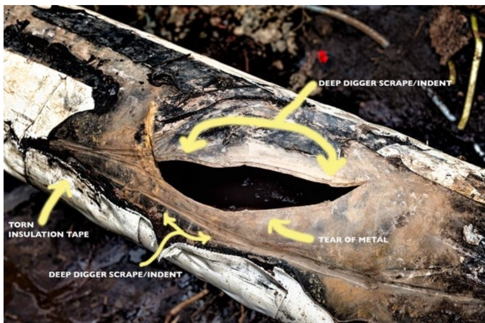
Figure 8: Photograph showing the damage to the pipeline
